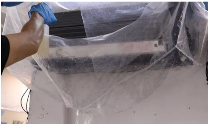
4. 安裝冷氣機污水收集袋以及噴上澳洲環保清潔劑 Multi-Enzyme HVAC Coil Cleaner
